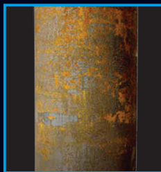
Top Competitor's Glass-lined Tank Very Heavy
